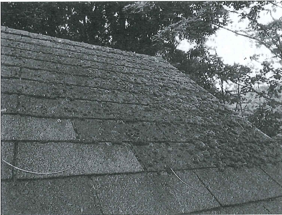
Photograph #16 - Moss Growth On Duplex Building
