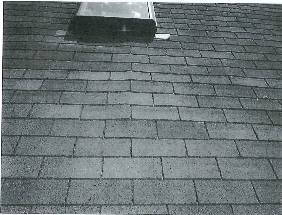
Photograph #14 - Plywood Decking Lifting
