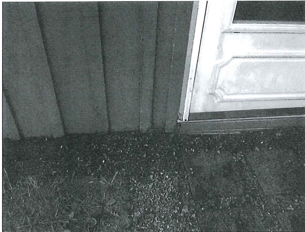
Photograph #8 - Deteriorated Siding On Triplex Building
