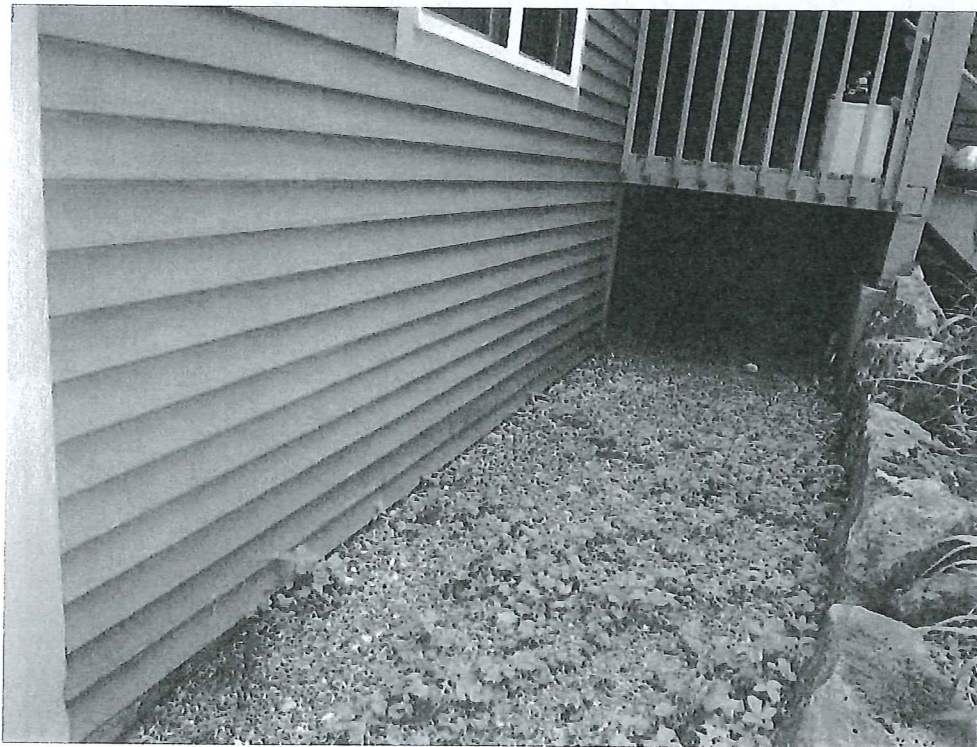
Photograph #10 - Siding In Contact With Grade Materials
