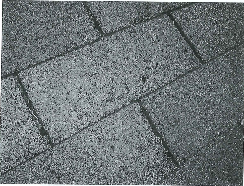
Photograph #13 - Blistered Roof Shingles
