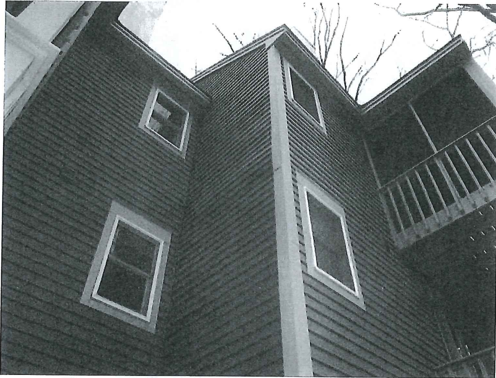
Photograph #9 - Bulging Siding On Rear Of Building #7
