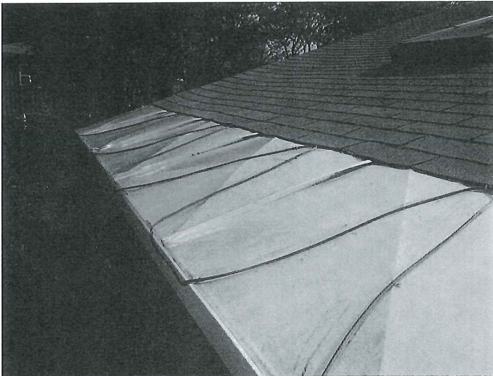
Photograph #12 - Metal Belt On Triplex Roof Eave
