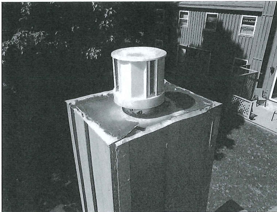
Photograph #20 - Triplex Chimney With Open Cap Flashing
