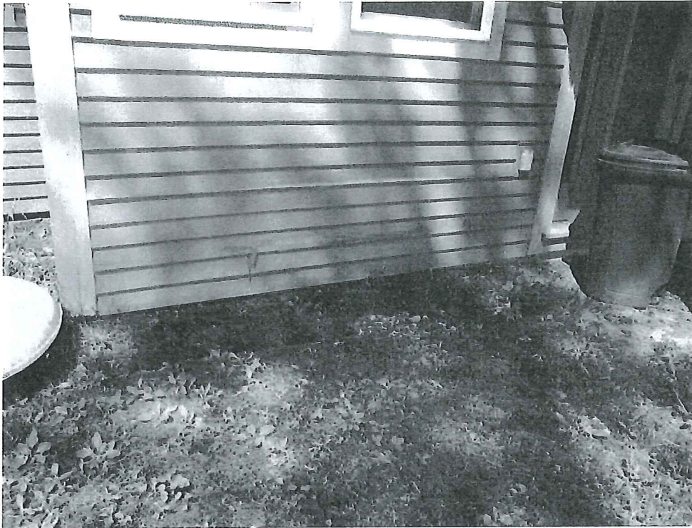
Photograph #11 - Failing Siding Finish
