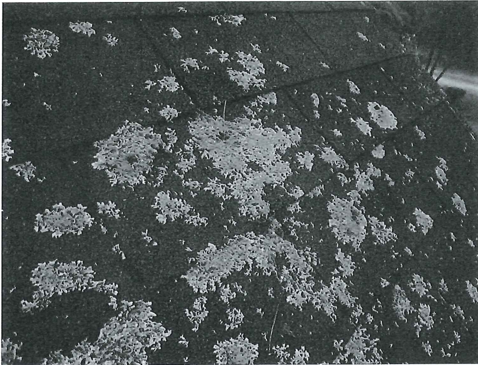
Photograph #15 - Lichen Growth On Duplex Building
