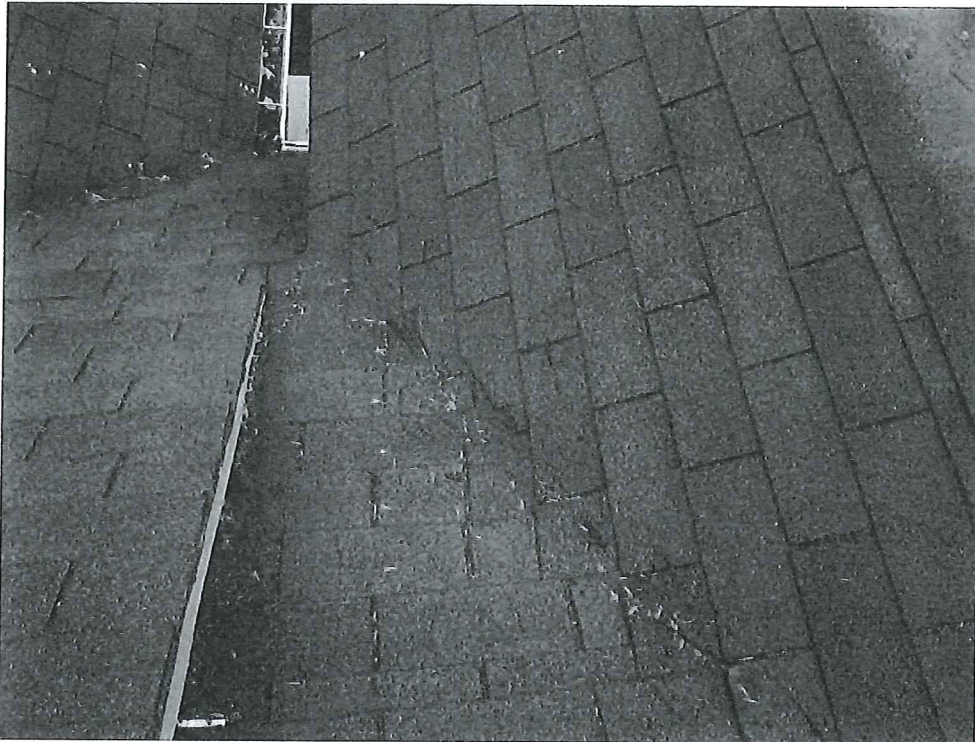
Photograph #17 - Damaged Roof Shingles On Duplex Building
